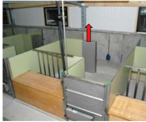
FAT 2 pens with earth heat exchanger
